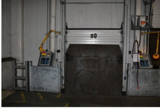
Figure 3. Bay 80 Subject Dock Leveler in Vertical Position
